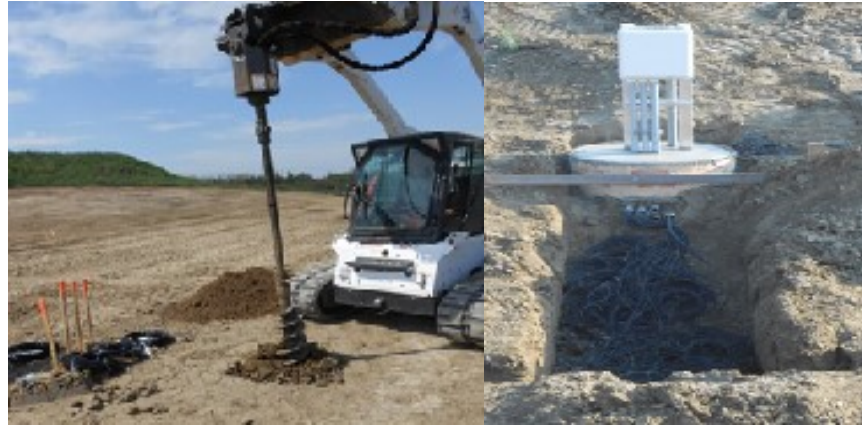
Figure 3-5: Installing the deep sensors using an auger (left); sensors' lead conveyed to the datalogger box in a trench (right)
