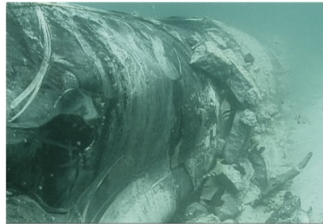
(b) Dent and rupture (offshore pipeline)
