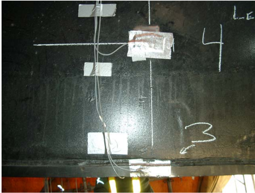
Figure 4 – Strain Gauge Installation on Web and Bottom Flange of Boom at Section A-A
