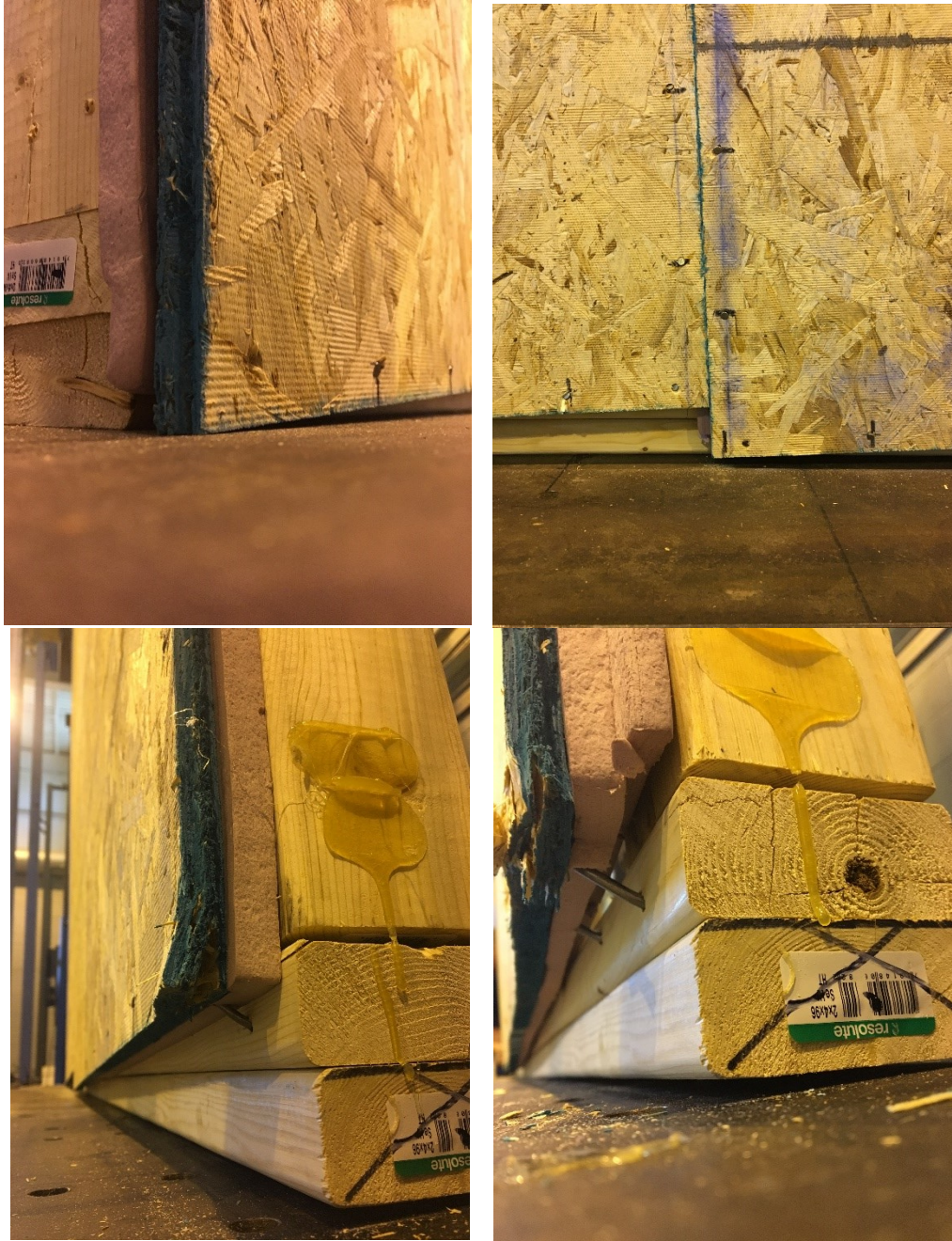
Figure D.2: Failure mode of S2, S3, and S4 Shear wall: nail bending
