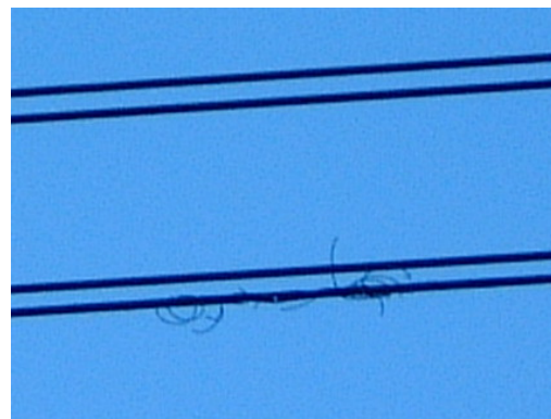
(b) Example of a conductor defect on a high voltage transmission line.
