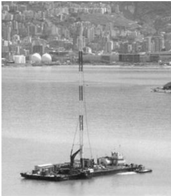
Figure 9. Installation of vertical drains by an installation rig mounted on a floating pontoon during the Beirut Project.
