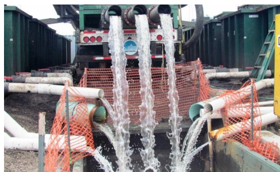
Figure 6. Clear Water Discharge from an AquaScreen and TerraCores.
