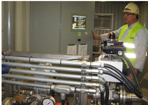
Figure 2. Polymer Injection System.
