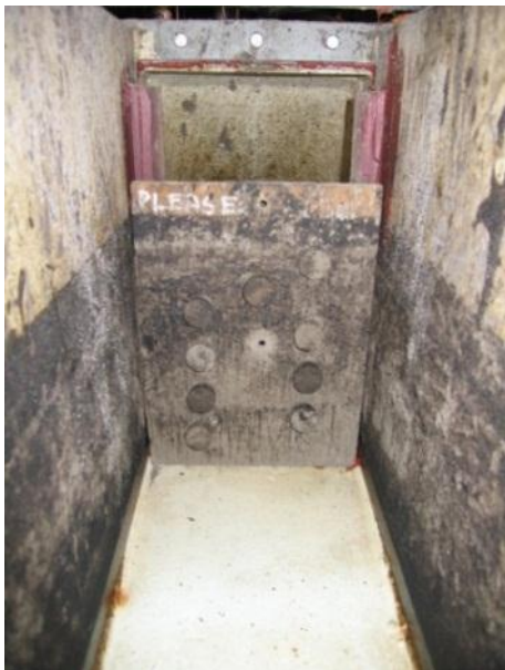
Figure 5. Rubber Plugs on Weir Board at Flume End.
