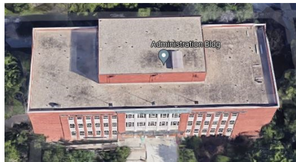
Figure 2. Google's 3D model of the ADMIN building. Imagery ©2021 Google, Imagery ©2021 Maxar Technologies, Map data ©2021
