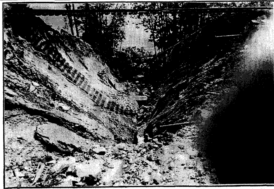
Figure 2-13 embankment overland flow erosion at MP 154.44, looking west (Canadian Pacific Railway, photograph taken in July 1998)
