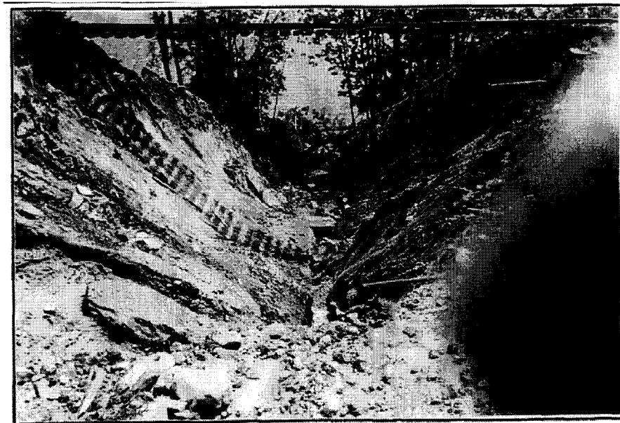
Figure 1-4 Complete overland flow erosion of railway embankment at MP 154.44 (from Canadian Pacific Railway, photograph taken in July 1998)
