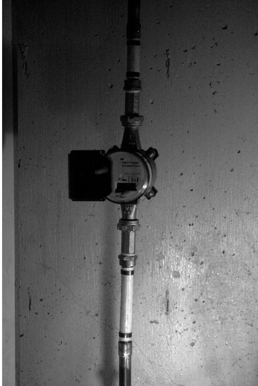
Figure 3.6 Installed and functioning water meter
