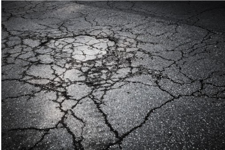
Figure 2-2: Cracks in Pavement [37]
