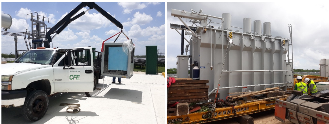
Figure 1.2. Delivery of a 45-kVA 1.2-ton auxiliary transformer (left) and a 40-MVA 38-ton step-up transformer (right) for a PV power plant (photographs taken by author).
