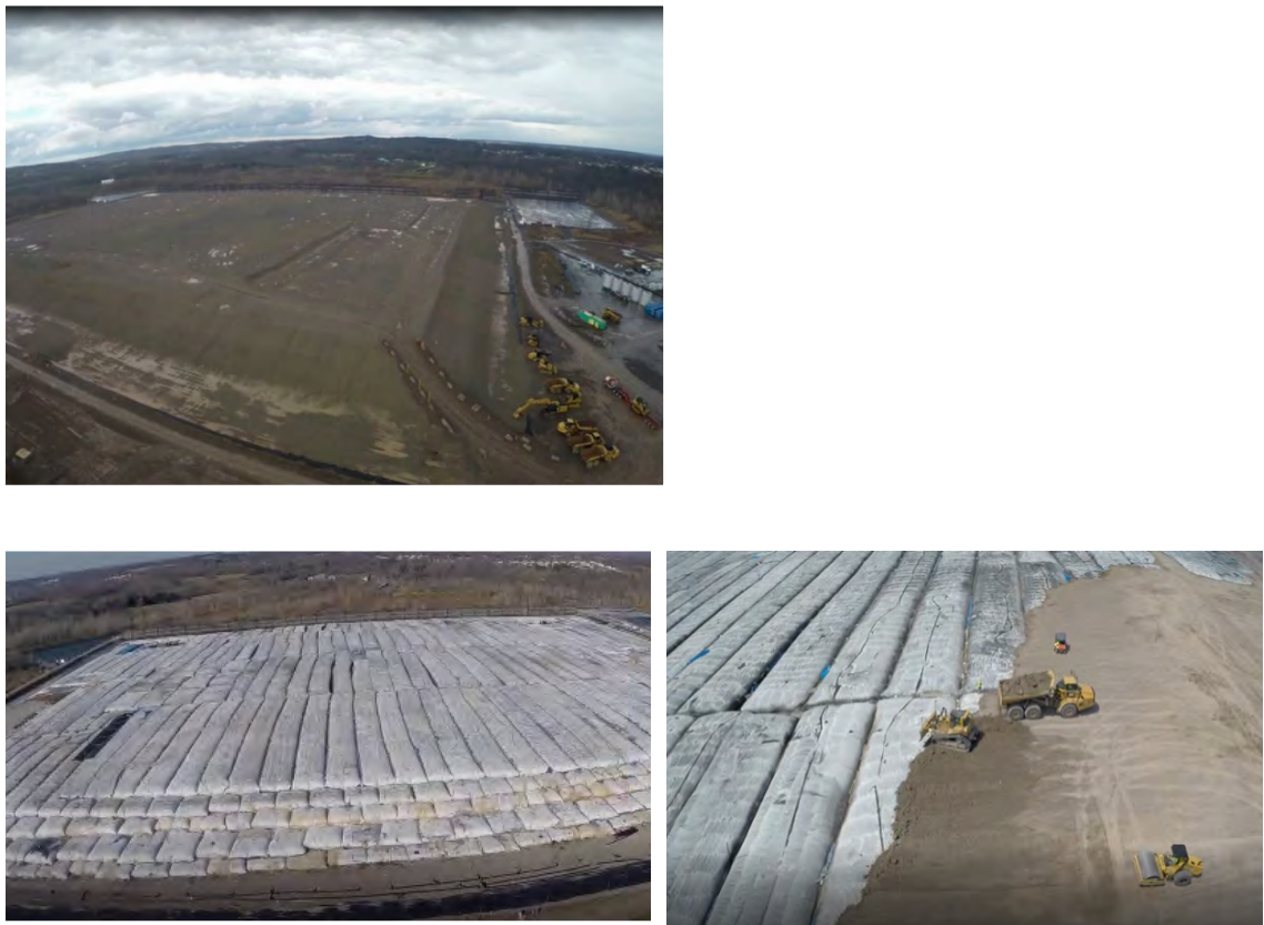
Figure 1-2: Example of stacked, capped, and reclaimed geotextile tubes deposit ~3MT/year (adapted from TenCate Geosynthetic Americas deposit of dredged limestone sediments).
