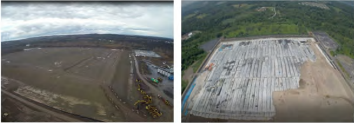
Photograph 4-18: Example of stacked geotextile tubes capped and reclaimed (adapted from TenCate Geosynthetic Americas).
