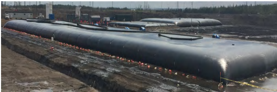
Photograph 4-15: Geotextile field trial with commercial tubes with size of 100 m length and circumference of 44 m.
