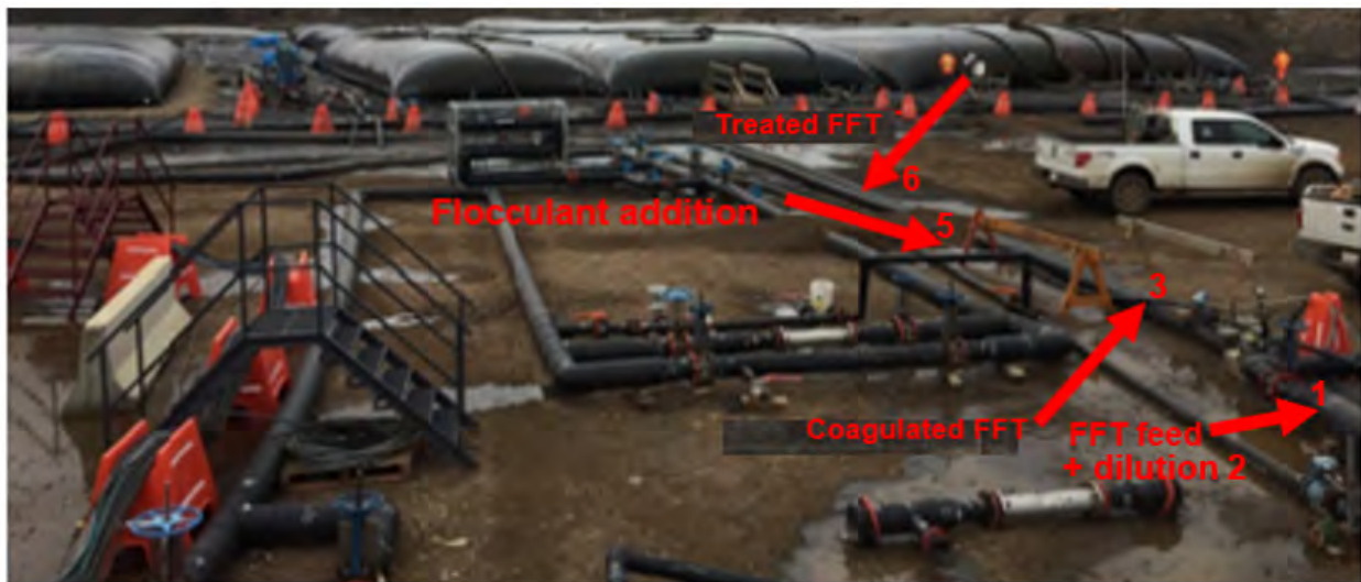
Photograph 4-11: Geotextile tubes field trial inline mixing process layout, and location of the flocculant injection/addition.
