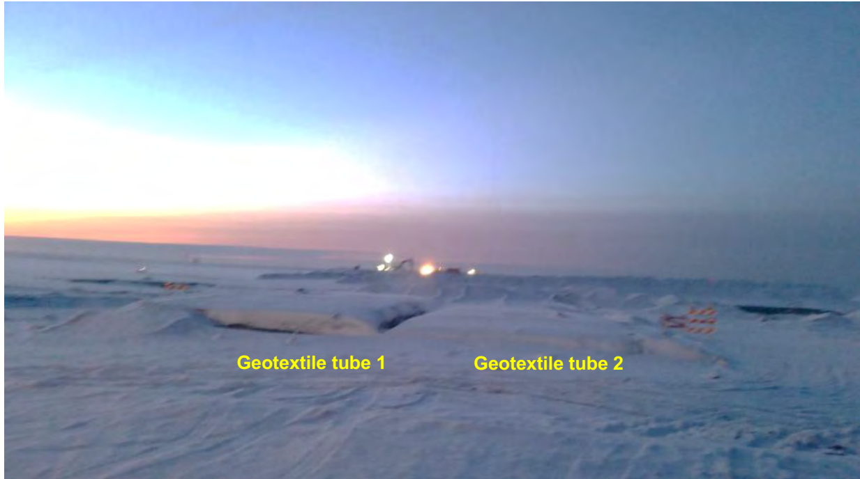
Photograph 4-10: Geotextile tubes trial after collecting the seven-day core sample (photograph taken on Dec. 5, 2014.)
