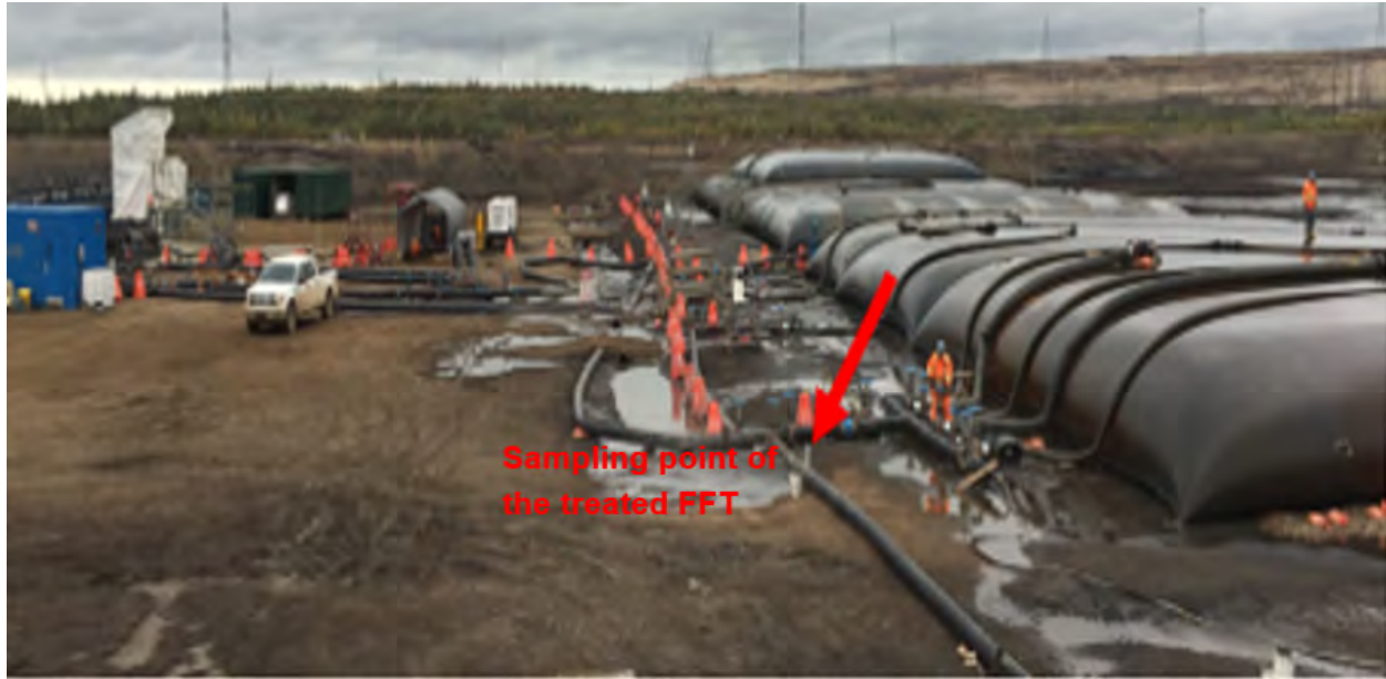
Photograph 4-12: Geotextile tubes field trial sampling location of the treated FFT prior to the discharge in the tubes.
