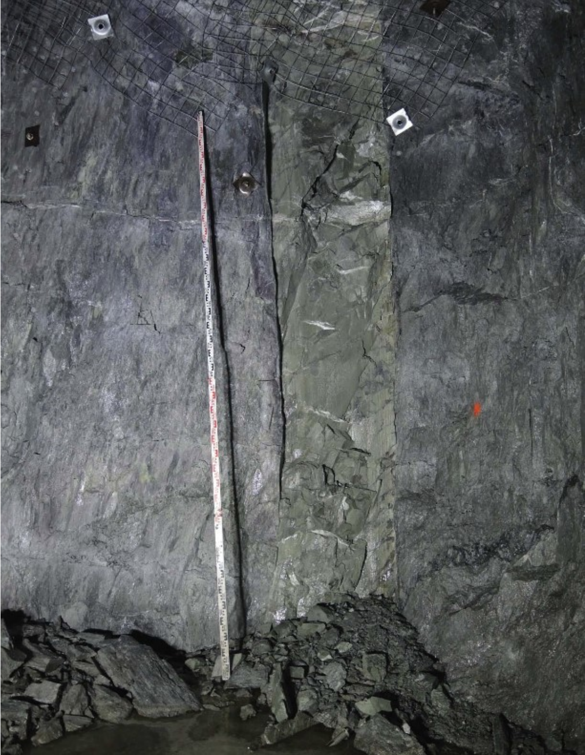
Figure 13 Trachybasaltic dyke showing subvertical nature (205/85W; underground location at 426664E, 6258158N, 1293m)
