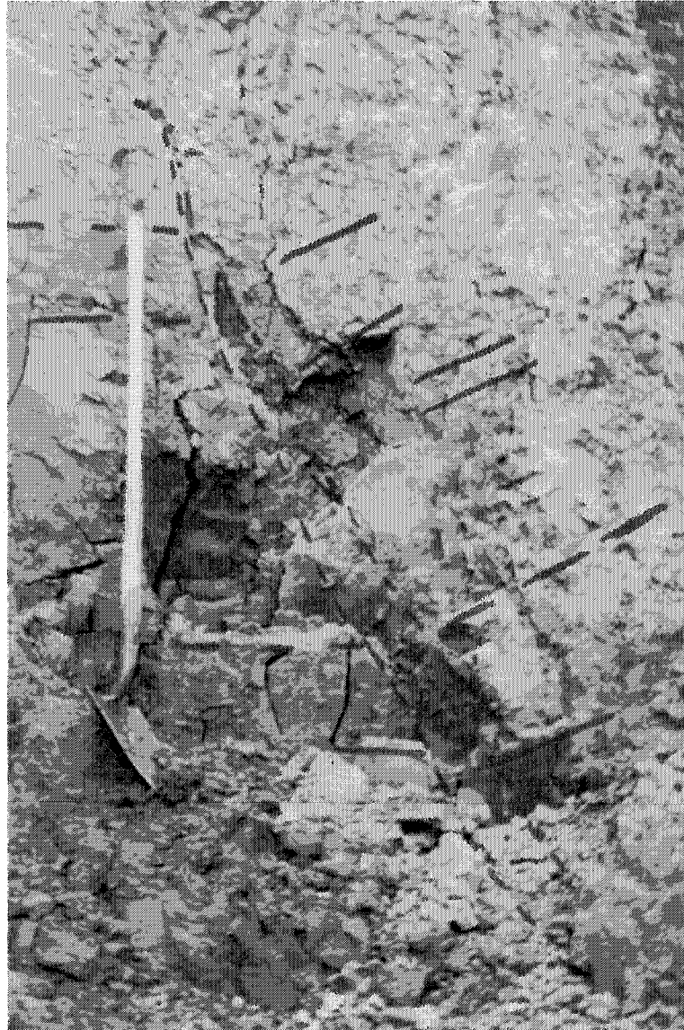
Figure 2.5 Excavation at the intersection of the main scarps of the prehistoric landslide and the 1993/1994 landslide (site 2 in Figure 2.2). Note the concave surface of rupture separating horizontal from rotated bedding. The horizontal bedding is undisturbed material outside of the prehistoric landslide. Shovel is 1.5 m long.
