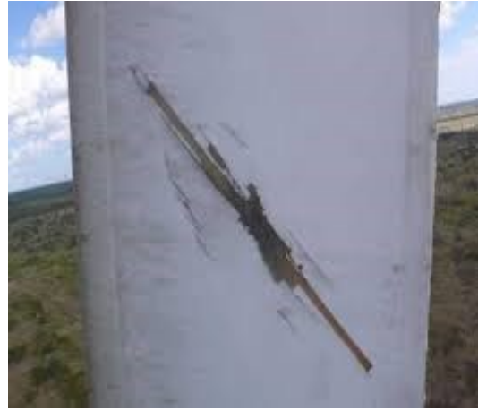
(b) lightning damage [8]
