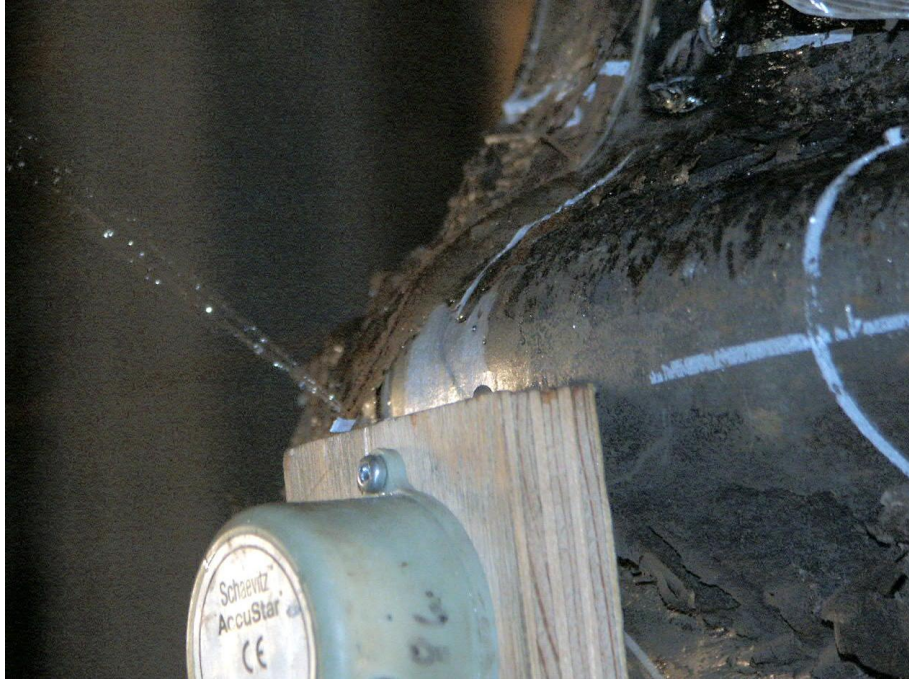
Figure 4.27: Pressurized water shooting out (LCF16N1)
