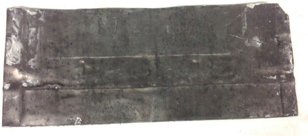
Figure 5-10 Failure of lead sleeve (bottom left)
