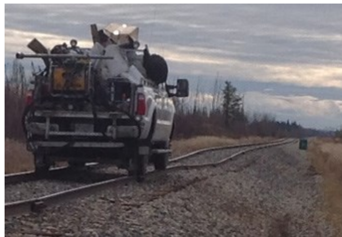
Figure 2-4. Excessive plastic deformation of a section of track constructed on muskeg
