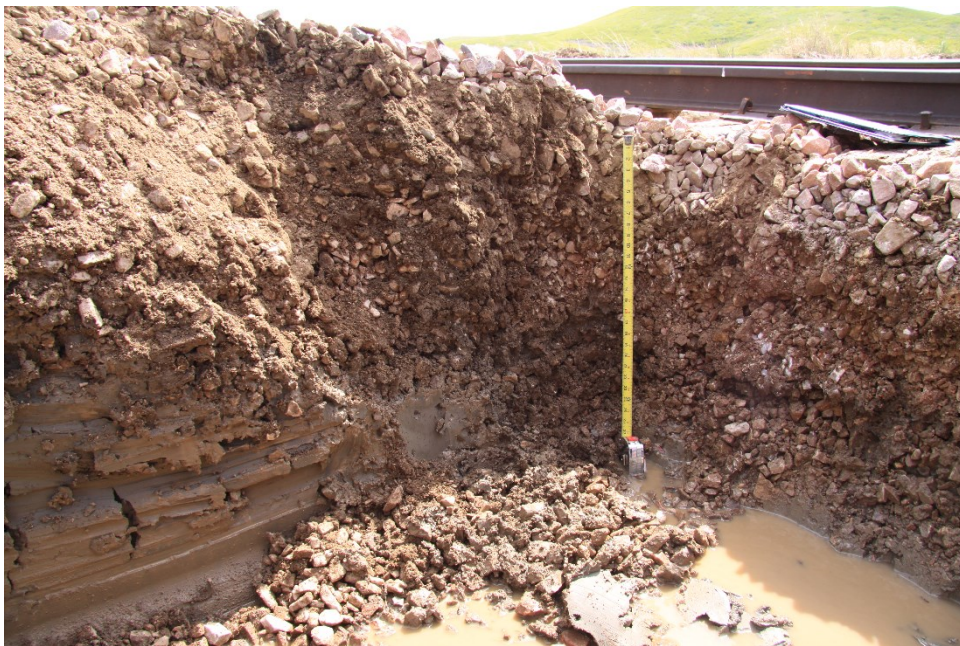
Figure 3-10. Photograph of one of five test pits, showing evidence of heave in the high plastic clays (left-hand side) and standing water at the base of the fill material.
