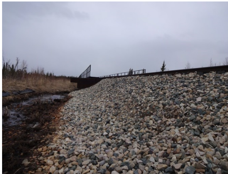
Figure A-3. High track embankment due to the cycles of track sinking and lifting
