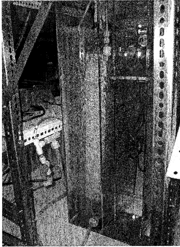
Figure 128. MBR2 membrane tank during the water test run.
