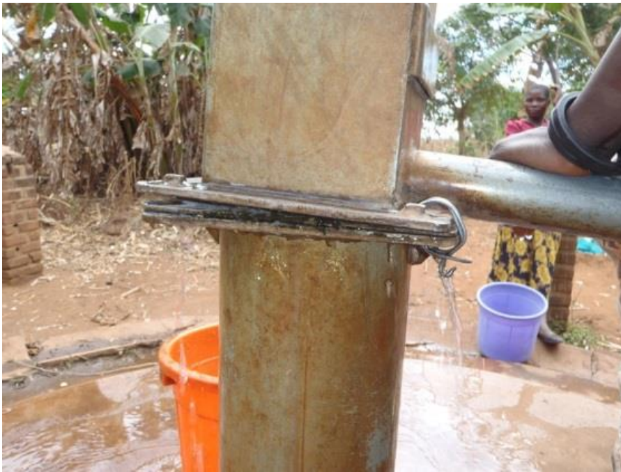
The absence of simple head-bolts can render a hand pump ineffective. This photograph shows a temporary fix while head-bolts were being sourced from Nkhoma (Kalonga Village)
