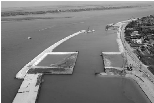
Figure 12. Malamocco Ship Lock
