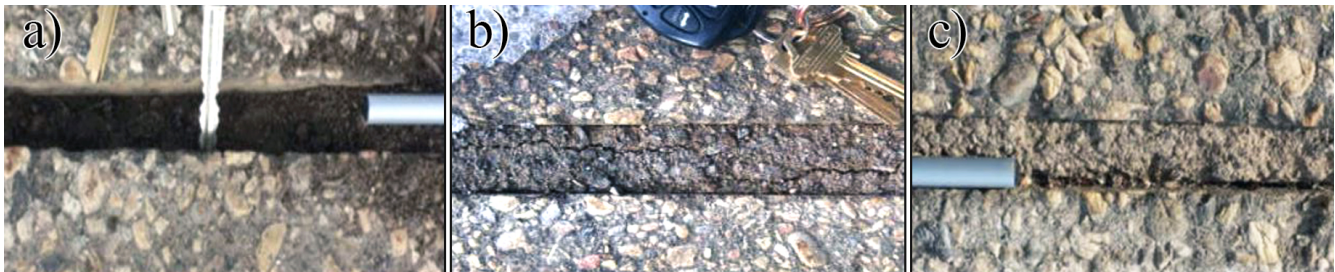
Fig. 2.4. Distresses of cold-mix asphalt in a micro-trench. (a) Backfilling settlement and cold-mix asphalt washed out, (b) lack of cohesion and (c) lack of bonding between cold-mix asphalt and the existing pavement [1].
