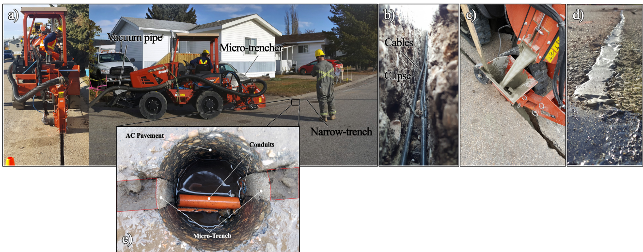
Fig. 4.1. Narrow-trenching using a micro-trencher. First a narrow-trench is cut (a), then the cables are laid at the bottom of the trench and secured in place by metallic clamps (b), and lastly, the cut is reinstated using a flowable fill (c). (d) shows the final reinstated trench. A cored section is also shown in (e).
