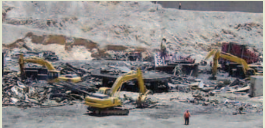
Barrick's use of advanced technology for building demolition at El Indio reduced safety risks and transferred skills to Chilean contractors.
