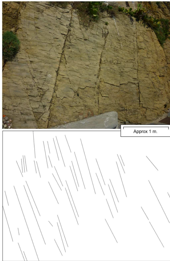
Figure 4.10: Above: An exposed rock face in Vernazza, Italy showing two fracture sets. Below: One of the fracture sets is digitized.
