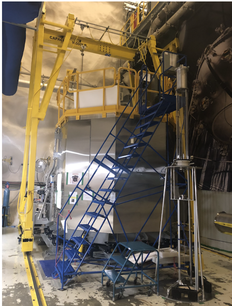
Figure 3.10: Fully assembled view of S140 as seen installed in the Cube Hall of SNOLAB during May 2022.
