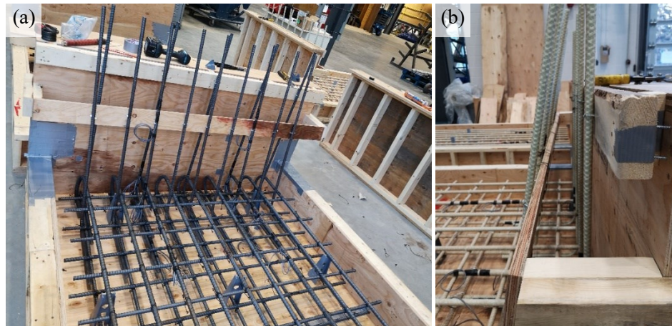
Figure A 1 Vertical reinforcement installation process for control specimens (a) front view of bars showing 2x4 in. sticks as guides, and (b) lateral view of wood guides used in SP-02.
