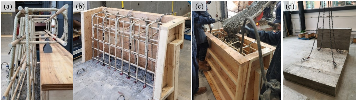
Figure 4.5 Barrier fabrication process for control specimens (SP-01 and SP-02). (a) barrier rebar assembly connected, (b) typical barrier formwork installed, (c) concrete pouring for barriers, and (d) formwork stripping after curing process finished.
