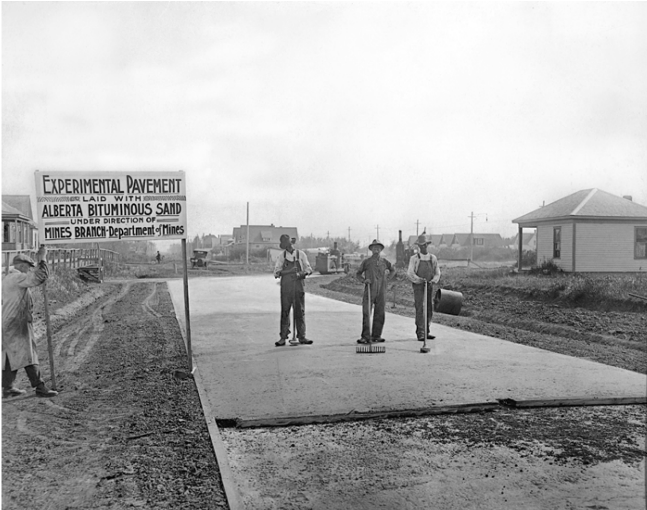
Fig. 23 Robert Fitzsimmons, Experimental Pavement Laid with Alberta Bituminous Sand under Direction of Mines Branch, Department of Mines.
