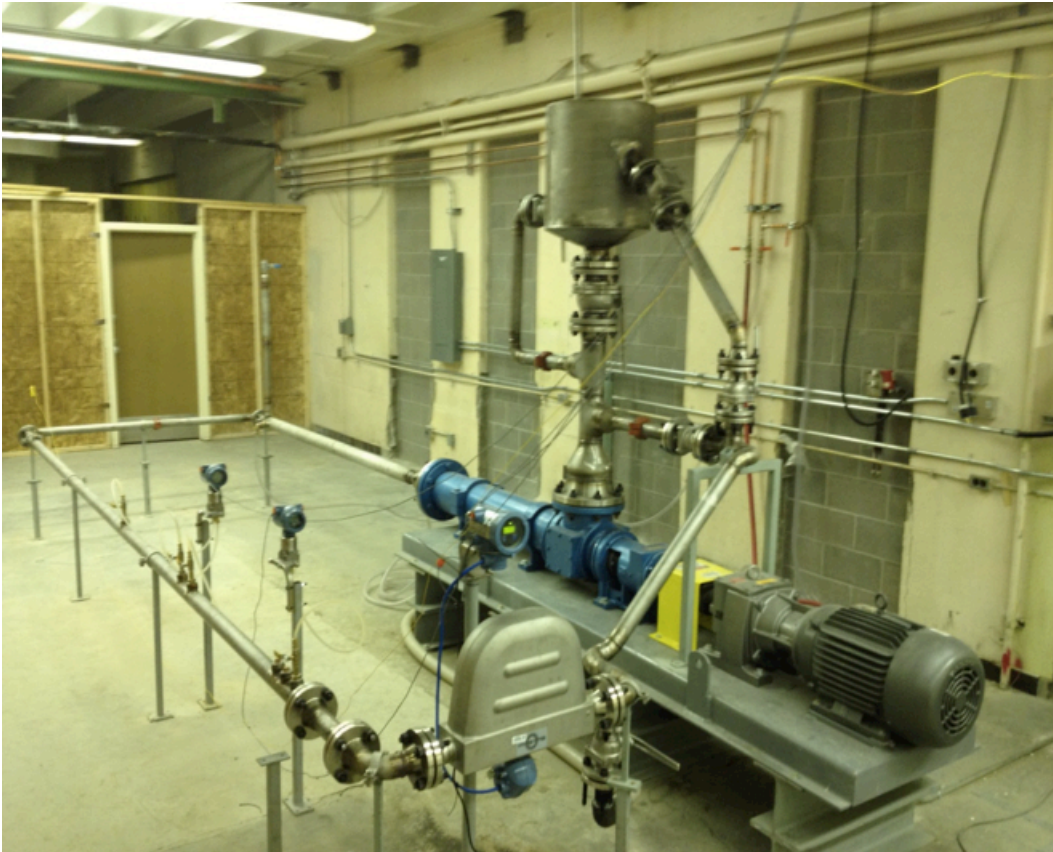
Figure 4.2 Photograph of the 50mm horizontal pipe loop used in experimental program
