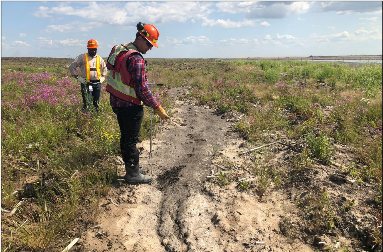
Photo 1. Crack near margin of soil placement area with cake (gray material) at the surface.
