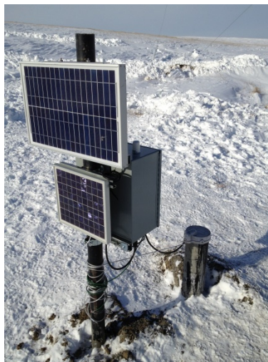
Figure 4-7: an individual radio unit contained within a completed tiltmeter station
