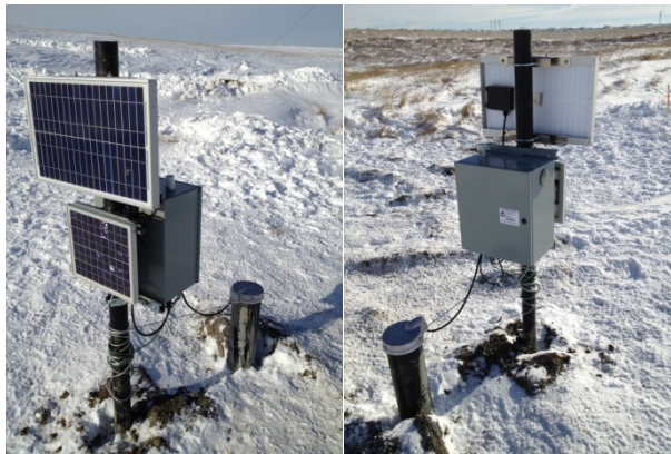
Figure A-7: Finished tiltmeter station
