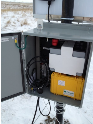
Figure 4-6: Tiltmeter station surface enclosure
