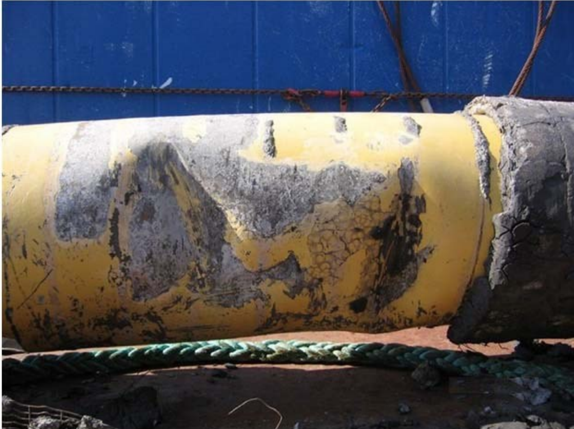
Figure 3 Photograph of kinked dent in field pipeline (Macdonald et.al. 2006)
