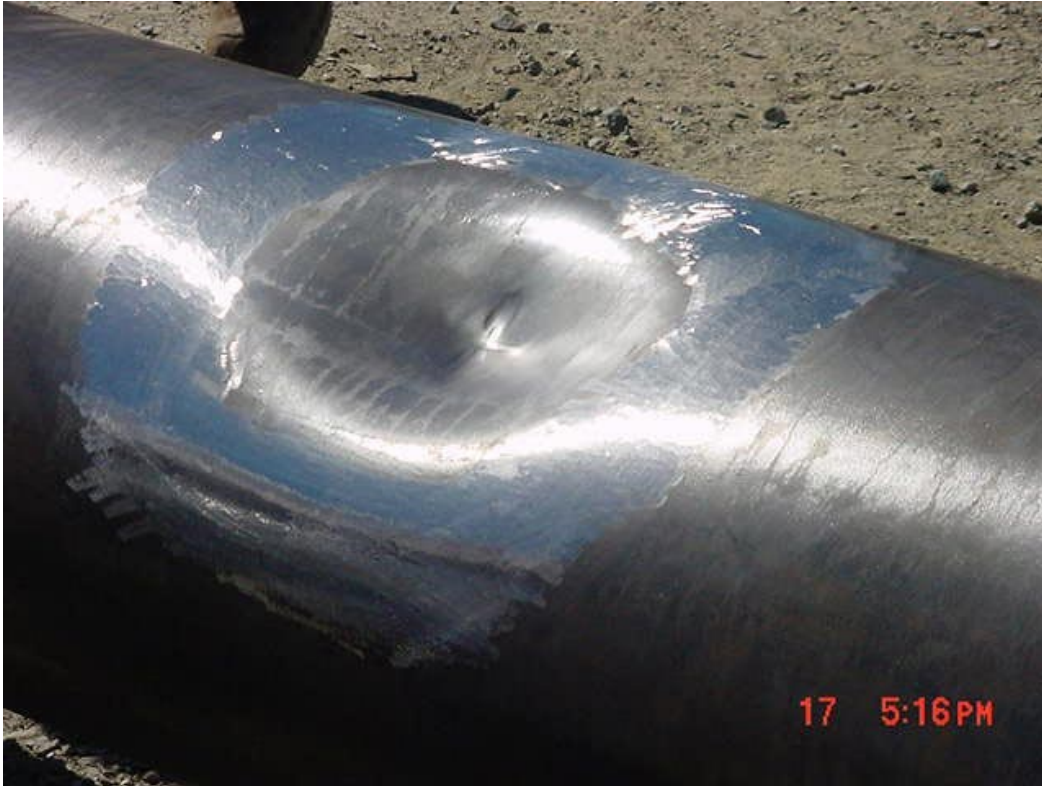
Figure 1 Photograph of a dent in the pipe wall (Source: http://www.google.ca/images )
