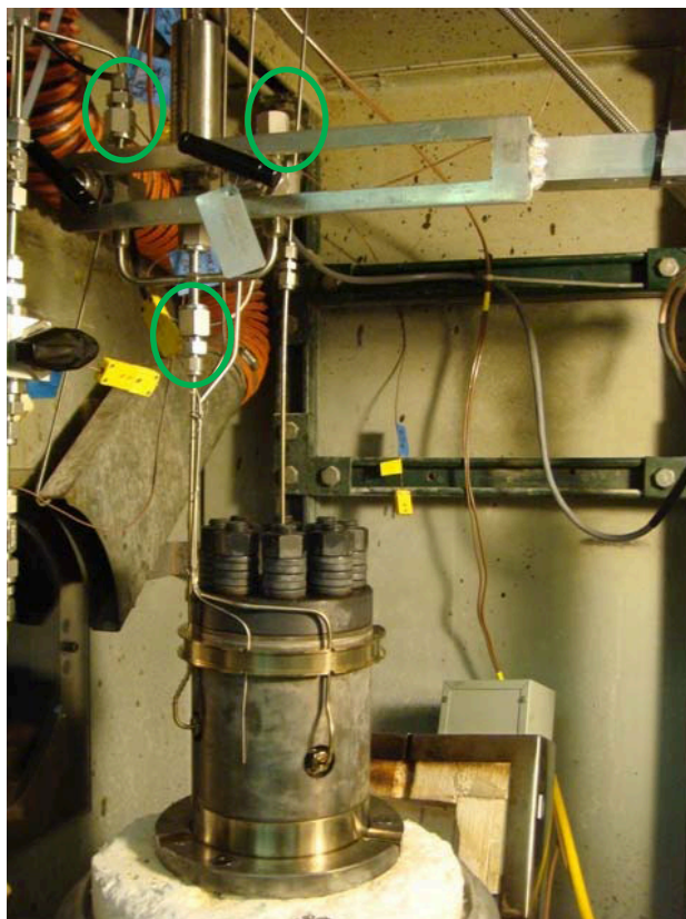
Fig A8: 3 VCR connections on the fork-shaped structure (specified by green circles)
