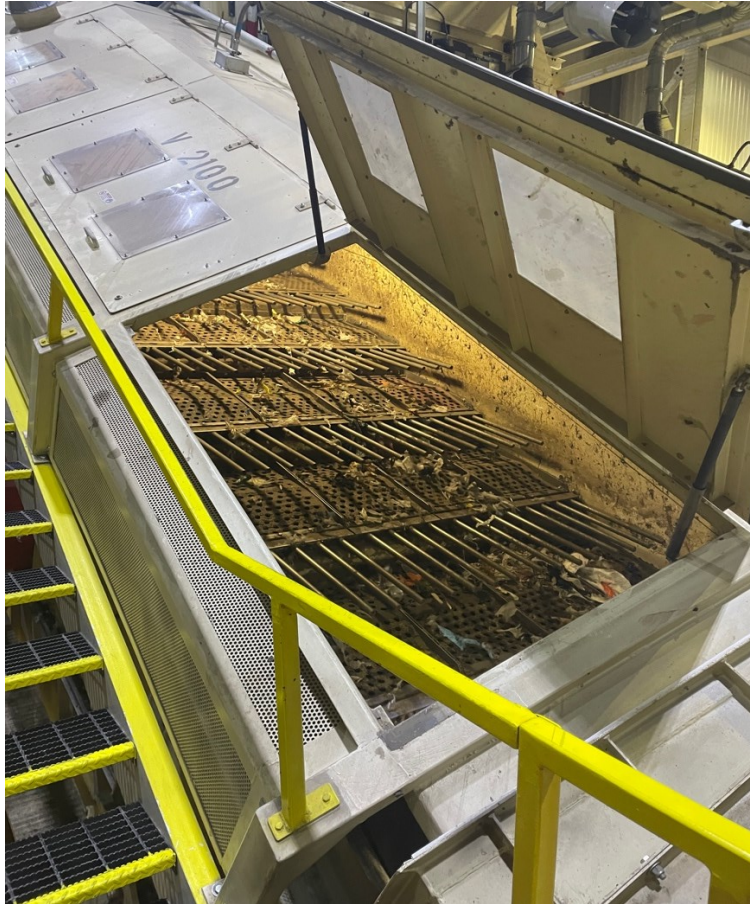
Figure 6: Inside the Waste Screen
