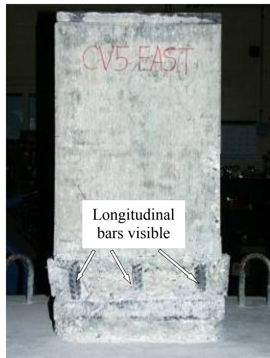
(h) At end of test (East side)
