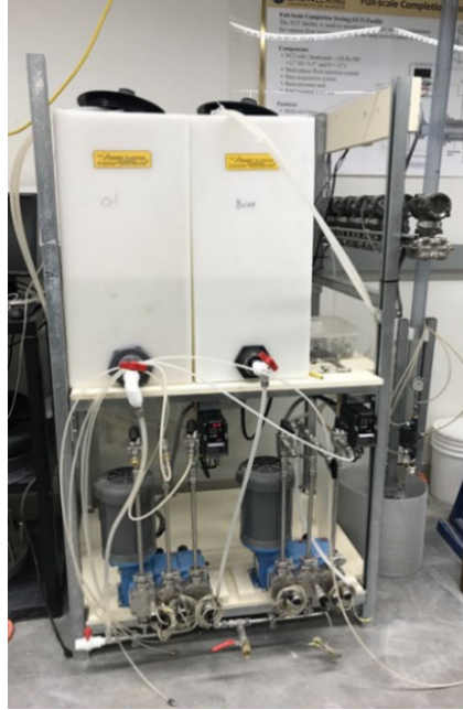
Figure 3-9. The photo illustration of the two triplex metering pumps
