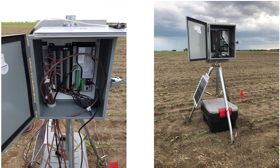
Figure A.8: Data logger, Multiplexer, Solar panel and Sensors
